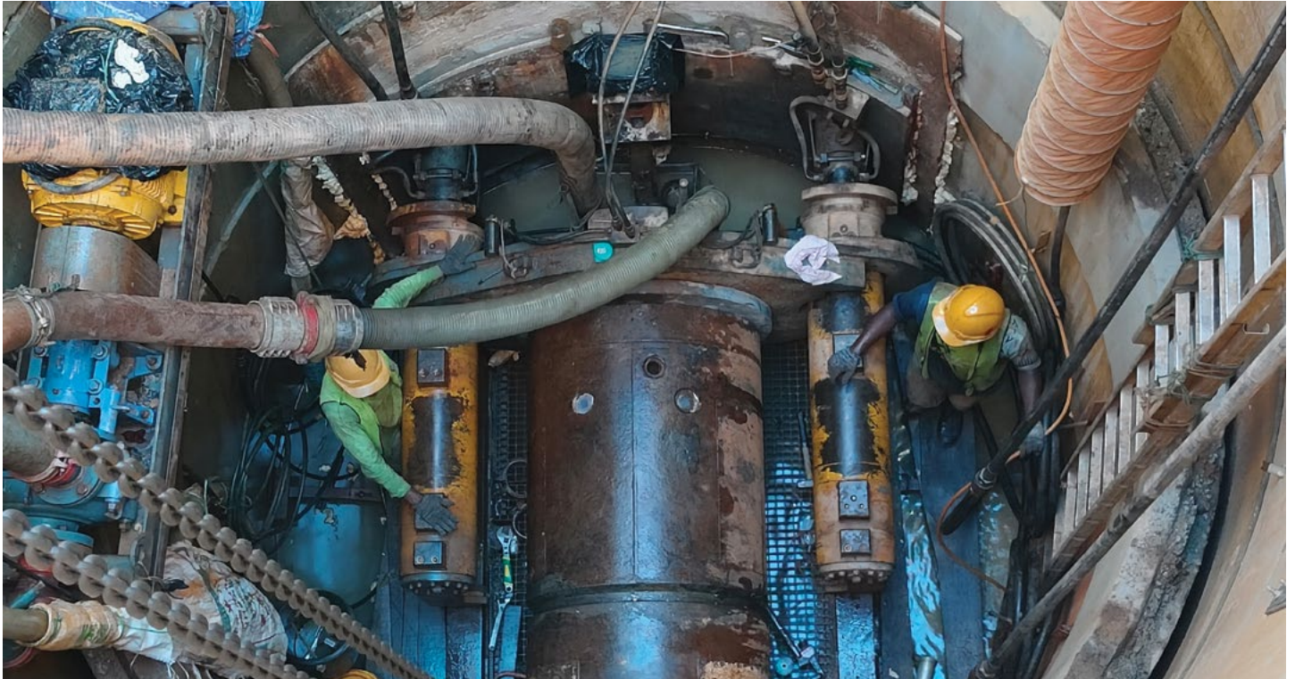
External Common Gravity Sewer Mains, Jalan Segambut
